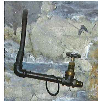
Repair of existing unsafe piping is exempted
