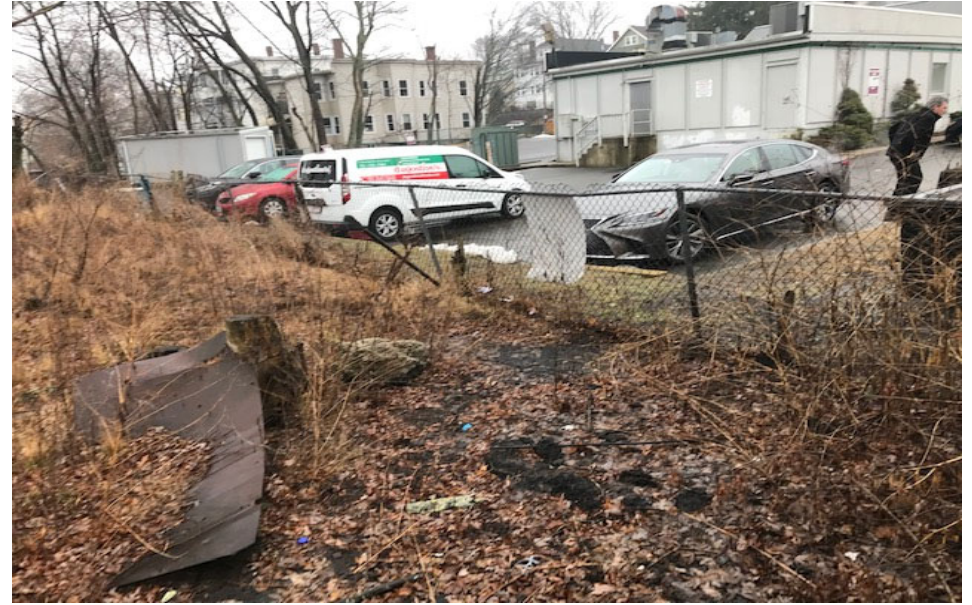
Figure 6: Eastern view of top of bank behind grease trap.
