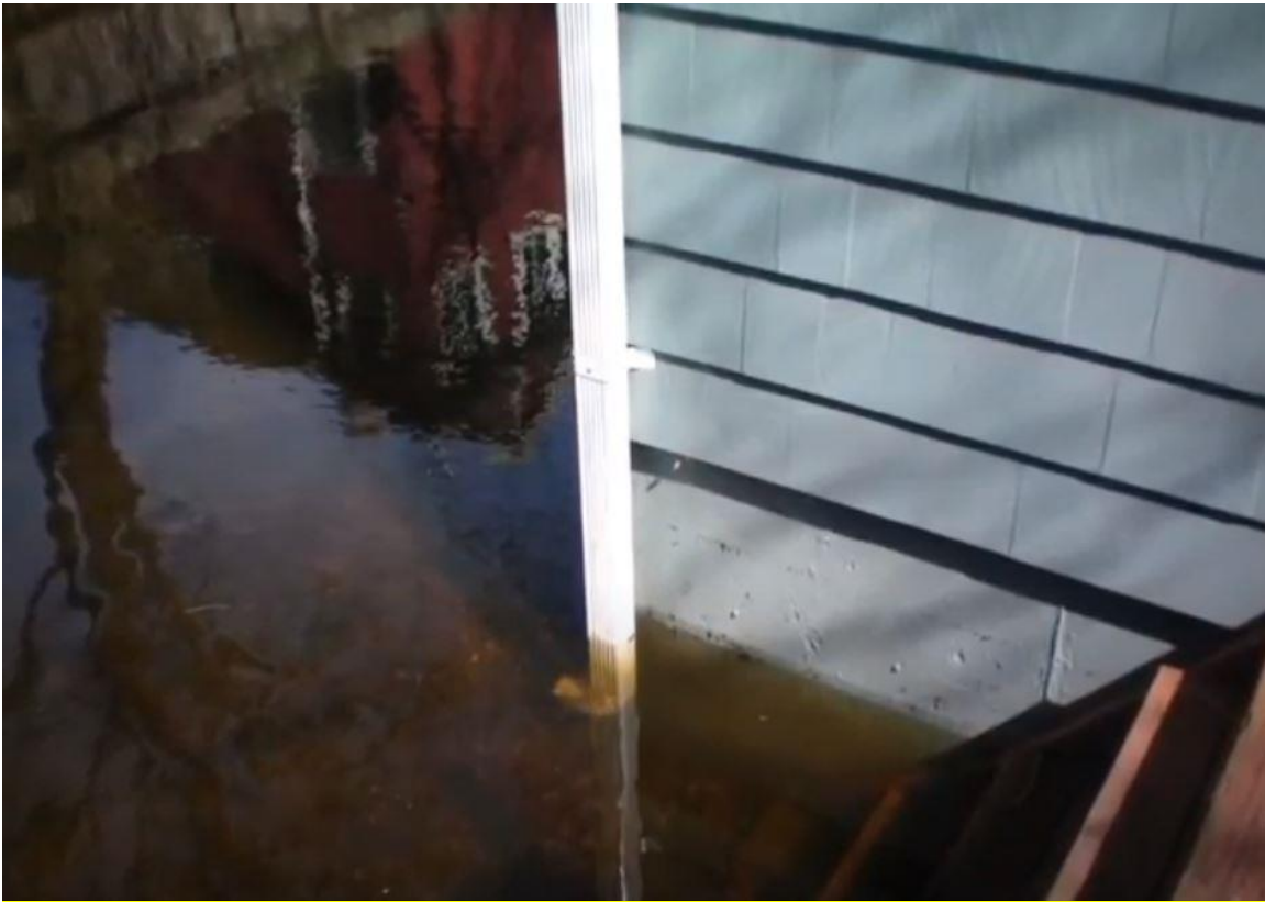
Figure 6. Flooding seen on Fairmont St. after 2010 storm
