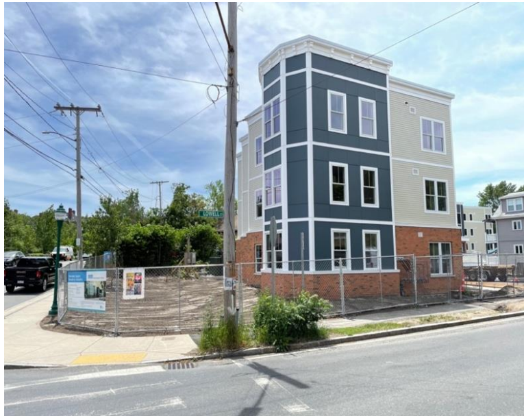
HCA's "Downing Square" affordable homes under construction, July 2021. (Photo by David Hagan.)
