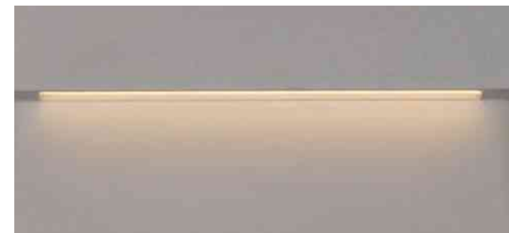
Recessed LED Downlight Grazers at Garage Screen
