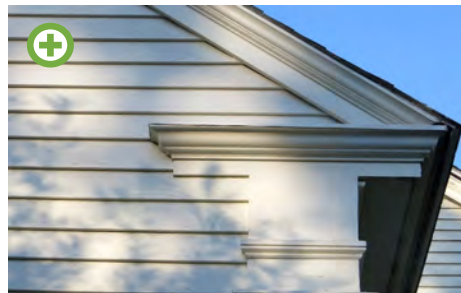
Example of a simple but effective eave return. (Source: This is Carpentry)
