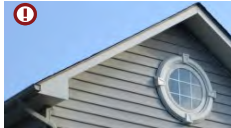
"Pork chop" eaves, steep return caps, or abrupt ends to the returns are less desirable details. (Source: This is Carpentry)
