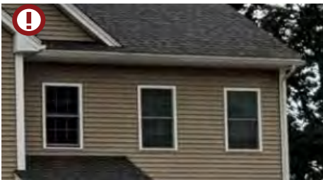
Gap between second-story windows and roofs. (Source: Google Streetview)
