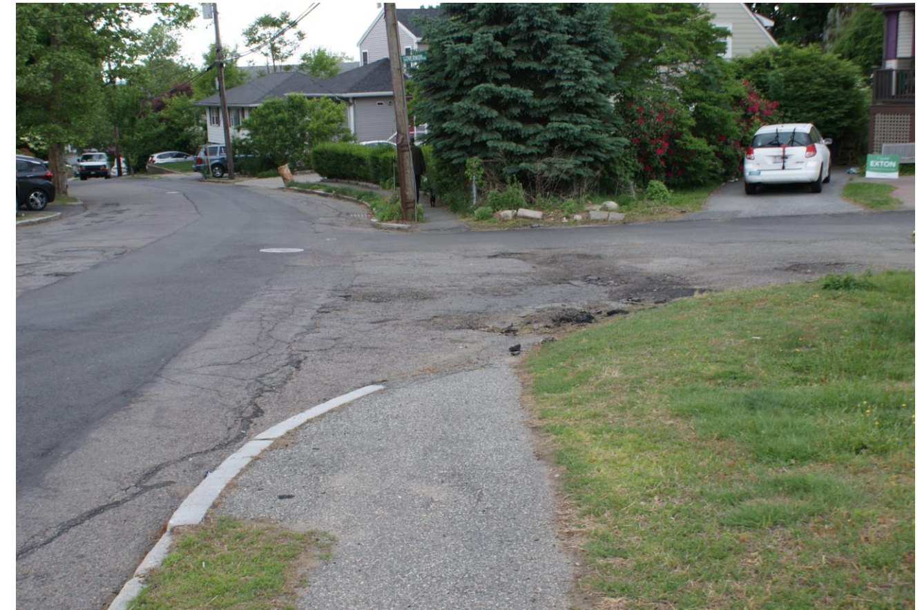
Missing crosswalks across side streets.
