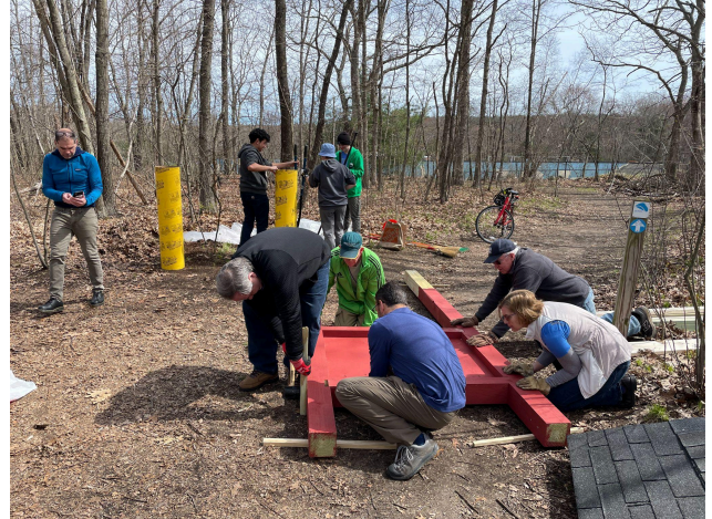
Helpers screwing the 6x6 posts, 4x6 cross beams, and plywood for the kiosk together while other helpers dig the holes for the 6x6 beams in the background.
