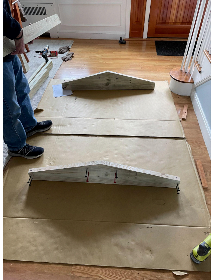
Setting up the ends of the roof and the screws to attach the 2x4 cross supports.
