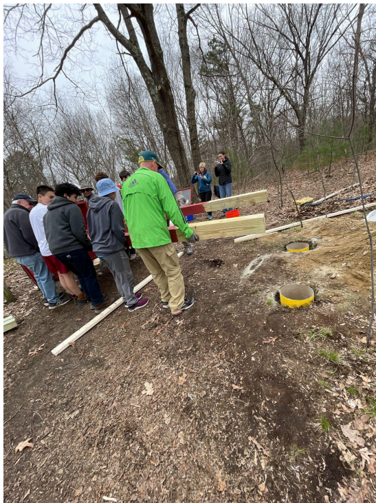
Picking up the kiosk to tilt it up into the holes with the concrete tubes in the ground.
