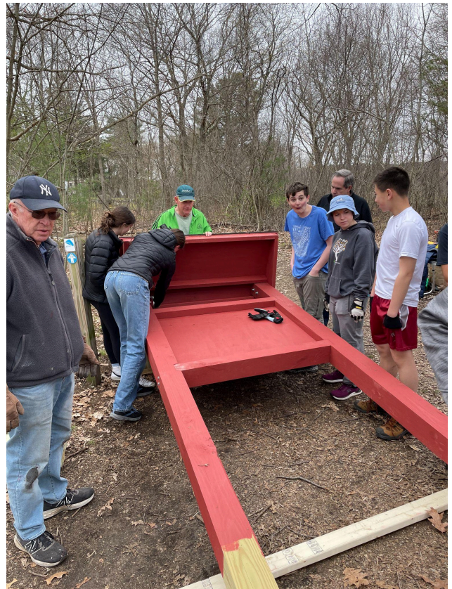
Attaching the roof to the kiosk on the ground before it is tilted upward into place.
