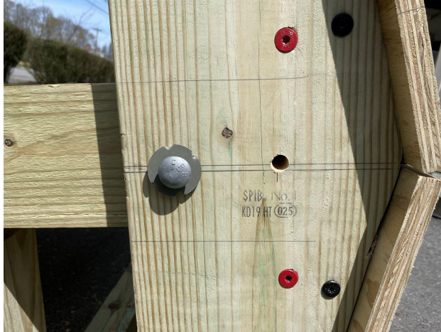
Drilled pilot holes for attaching the roof to the 6x6 posts of the kiosk.
