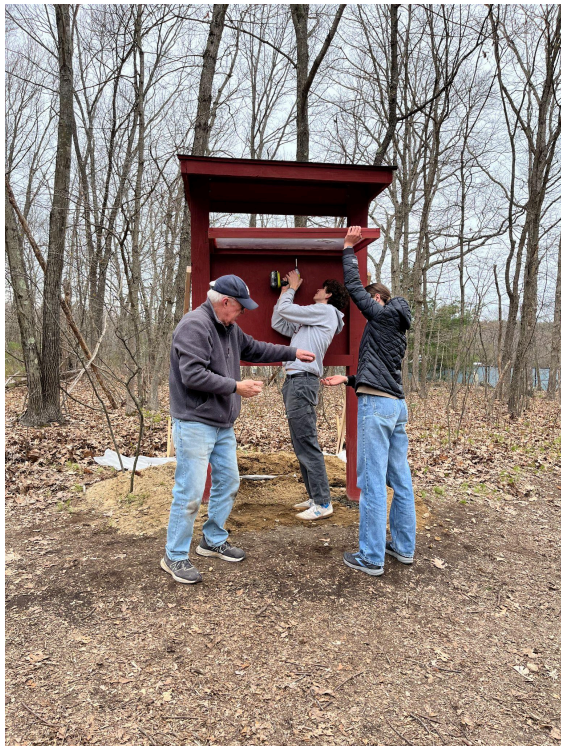
Screwing the hinged plastic covering into the topside of the information board.
