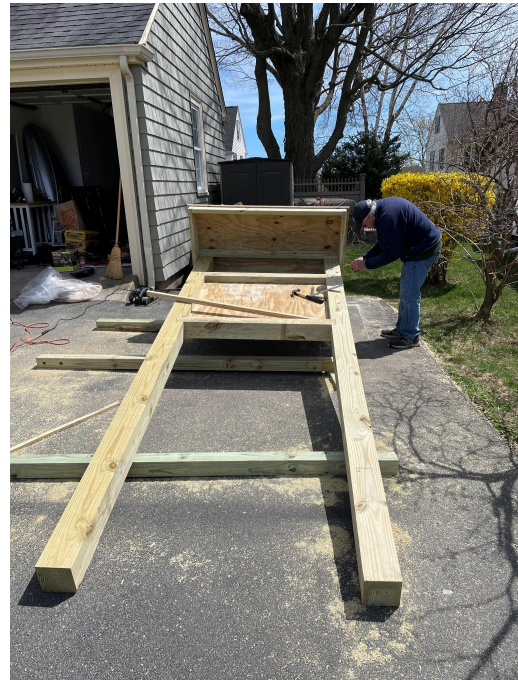
Assembling the kiosk in the driveway in order to drill pilot holes for attaching the roof and make sure the pieces fit together before the on site assembly.
