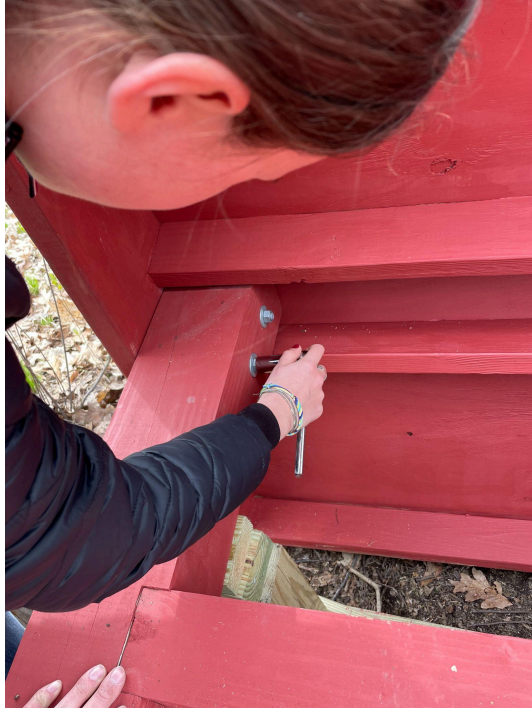
Tightening a nut on one of the carriage bolts that is holding the roof onto the 6x6 post.
