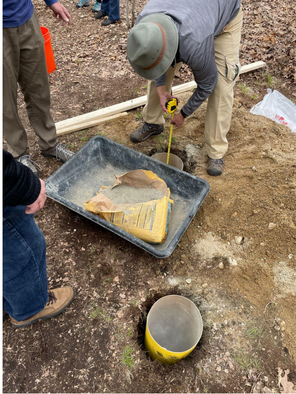
Mixing the concrete to pour into the holes once the posts were in them.
